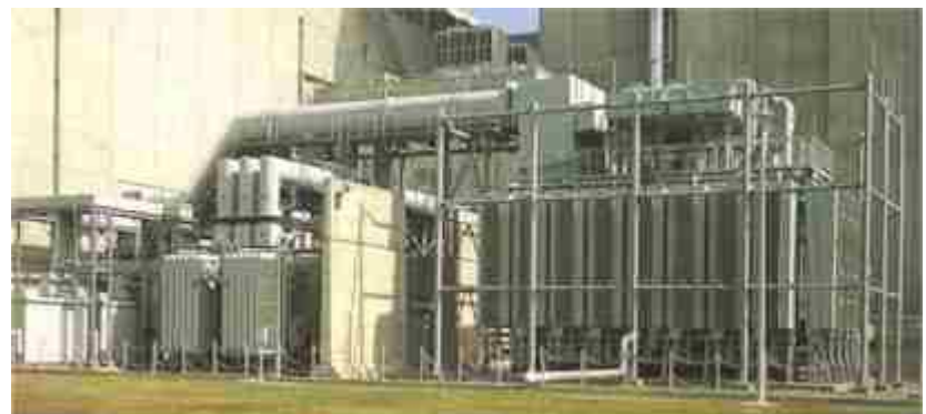
In operation at site
