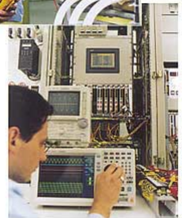
Site Tests Performance tests are carried out combining ● all controllers and protection devices and ● all AC and DC auxiliary equipment.
