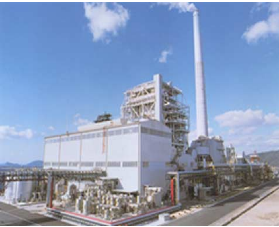
145MW Industrial Power Station
