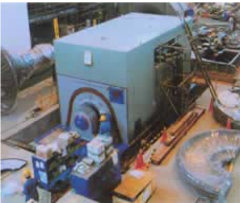
166MVA Air Cooled Generator
