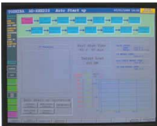
STATUS AND INSTRUCTION FOR TURBINE START-UP: TREND GRAPH ESSENTIAL FOR TURBINE START-UP OPERATION
