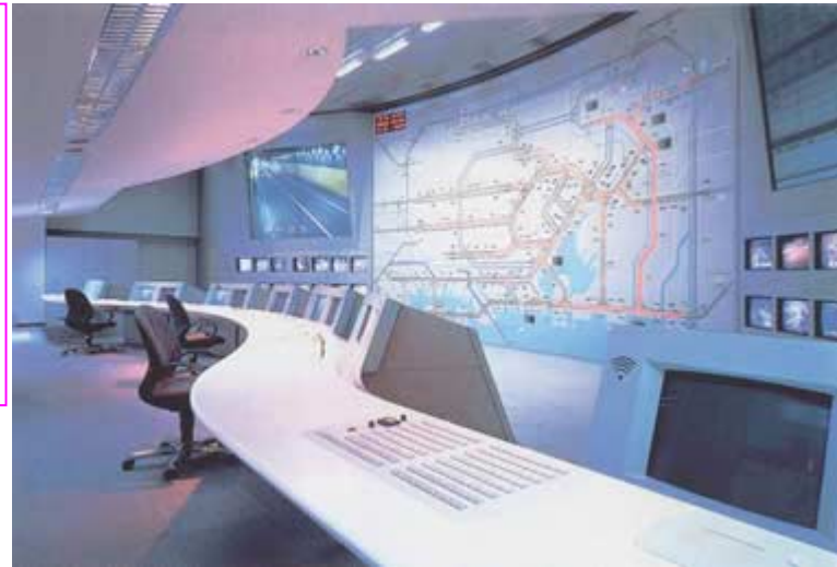
▲ Road traffic control systems
