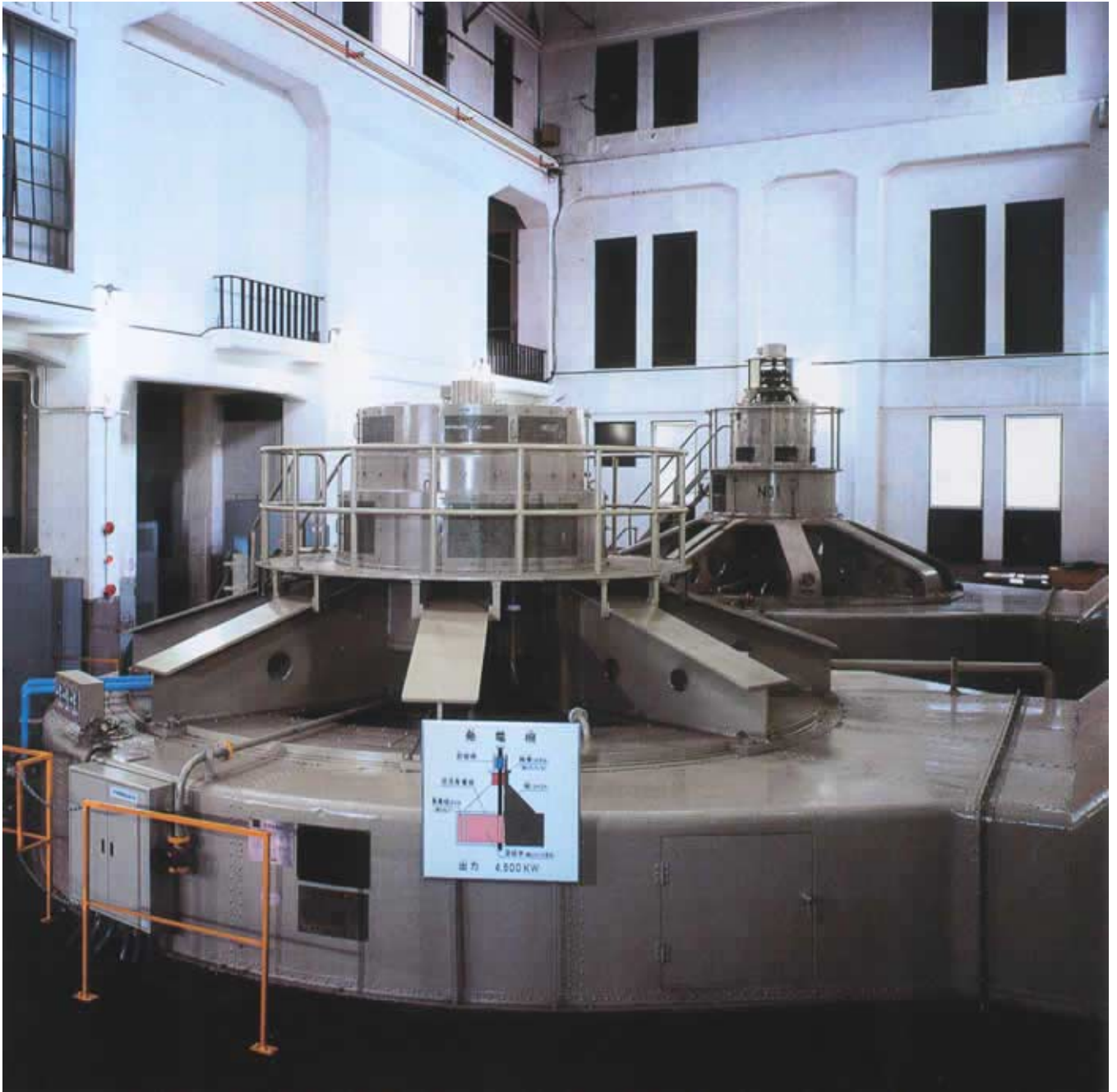
Example of Generator before Modification (Background) and after Modification (Foreground)
