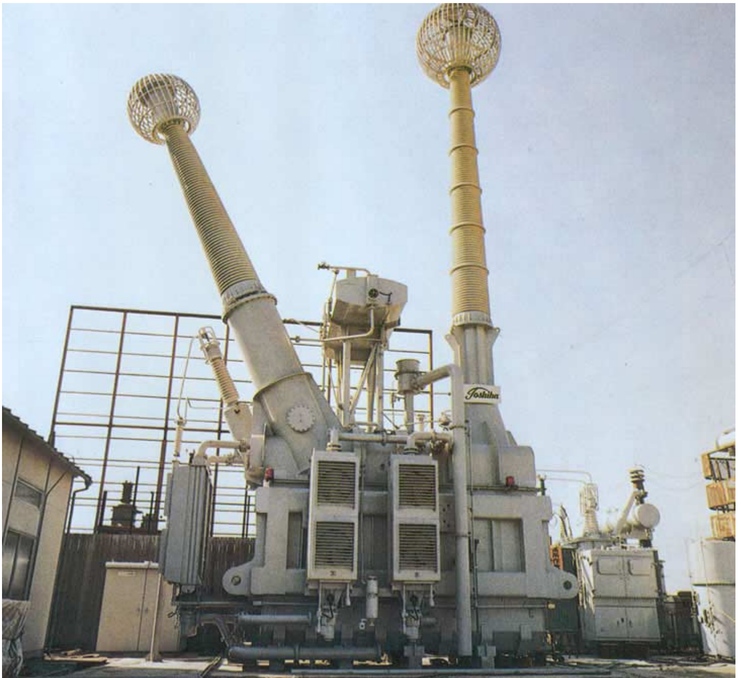
Fig.53 UHV Prototype Auto-transformer 500/3MVA-1200 \sqrt{3} kV-50Hz
