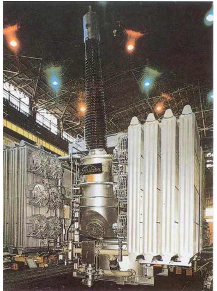
Fig.26 345kV-75MVA Forced-oil, Forced-air-cooled type Transformer
