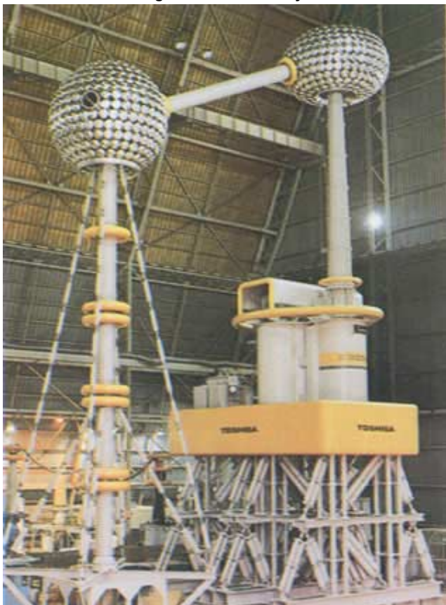
Fig.50 2300kV AC Testing Facilities
