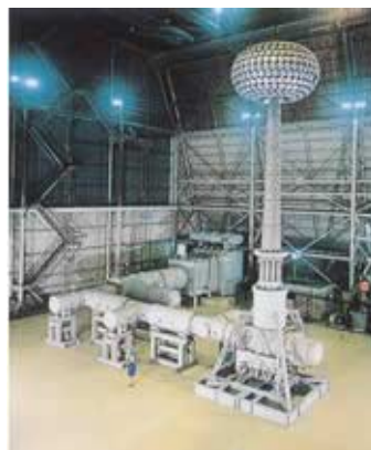
2,300kV AC Testing transformer
