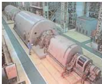
Short circuit generator
