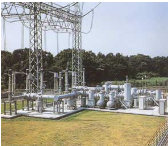
300kV GIS (All three phase encapsulated type)
