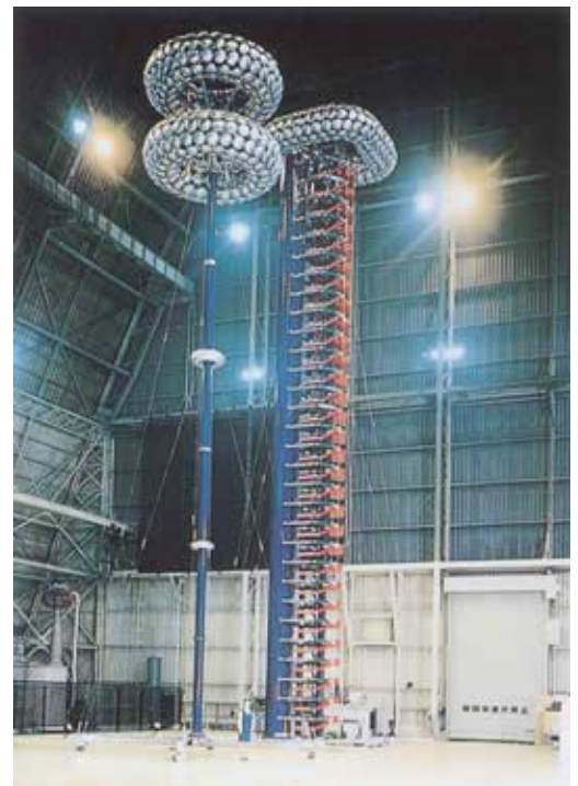
6,000kV Impulse generator
