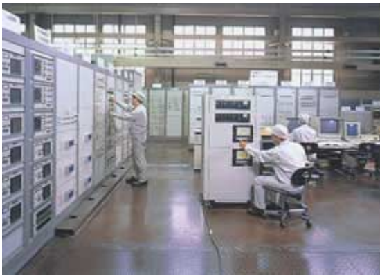
Power system simulator Performance of control and protection equipment is fully verified using the power system simulator.
