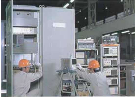
Control and protection equipment Control and protection equipment is tested individually.
