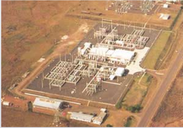
DC17.9Kv 50MW Fig.6
