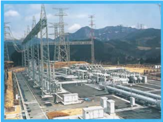
Toshiba has supplied a lot of switchgear covering voltages from 72kV to 1100kVAC. The picture shows 550kV Gas insulated switchgear with three phase encapsulated main busbar.
