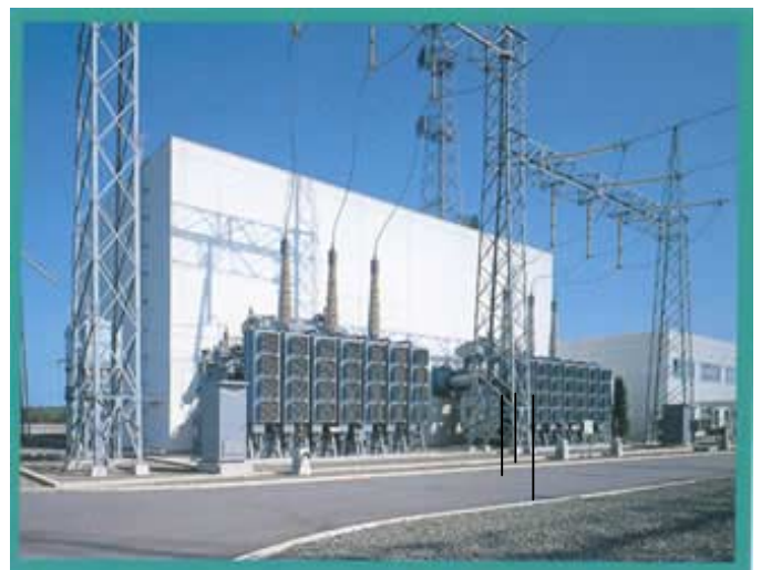
Toshiba has supplied many transformers up to 800kV since 1894. The picture shows converter transformers for an HVDC link.
