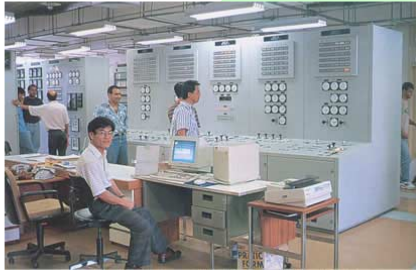
Site A performance test is carried out, •Combining all control and protection •Equipment with all AC and DC equipment
