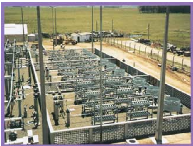
The picture shows an AC harmonic filter for an HVDC project.
