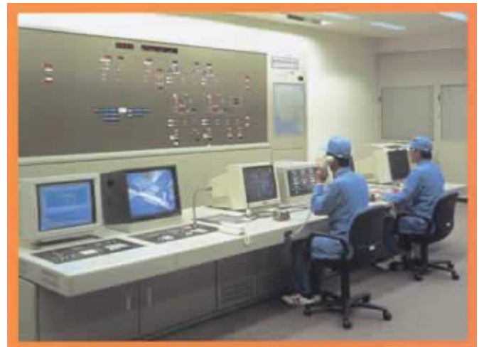
Toshiba produce telecontrol devices, man-machine devices, programmable controllers, power system controllers, converter controllers, and protection relays. The picture shows a supervisory control and data acquisition (SCADA) system.
