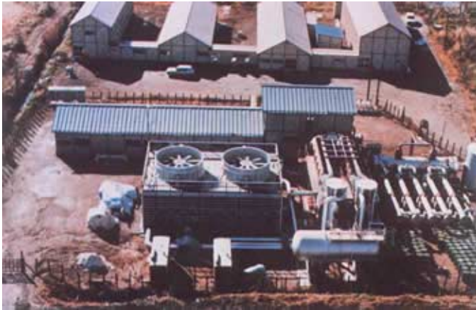
Nigorikawa Geothermal Power Plant Agency of Industrial Science and Technology, MITI, Japan 1 x 1000kW Binary cycle.
