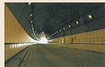
道路監視制御システム Monitoring and control system for road traffic
