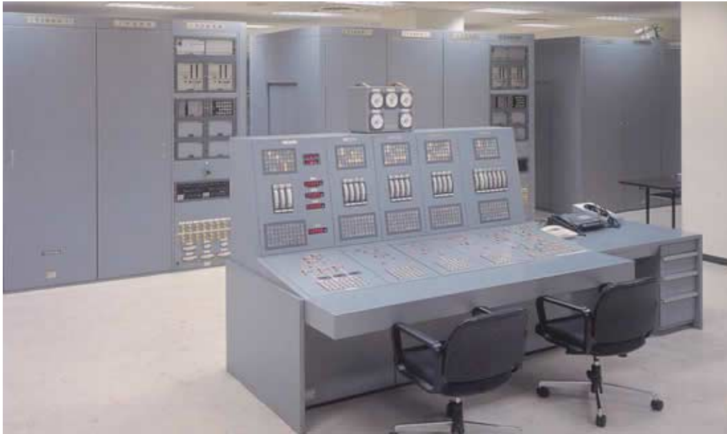
Unit Control board
